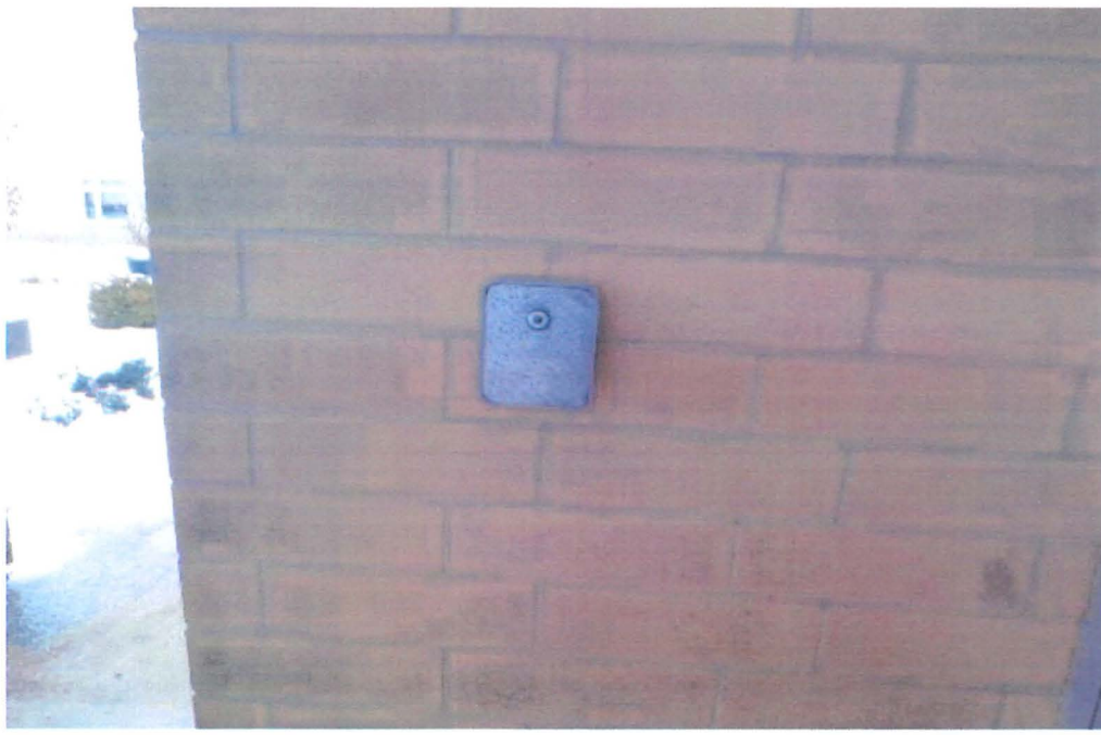
The key Lockbox for Fire Department access is located outside at the front entrance on the left wall.
